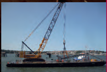
← Armed and ready - Williams rebuilt a massive crane on top of one of their barges in order to lift the giant loading arms off Valero's jetty for servicing.
