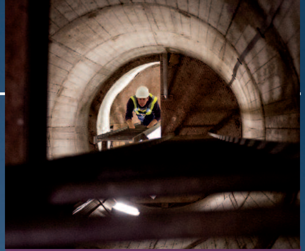
↑ Every bit of equipment needs regular maintenance. Here electrician Matthew Jones scales the 50m Watwick Tower to check the equipment.
